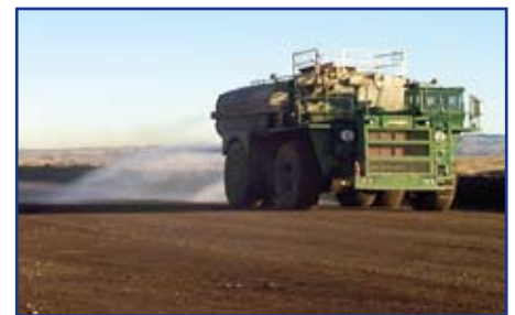
Dust Abatement with CBNG discharge water in the PRB. Photo Courtesy of Fidelity Exploration.
