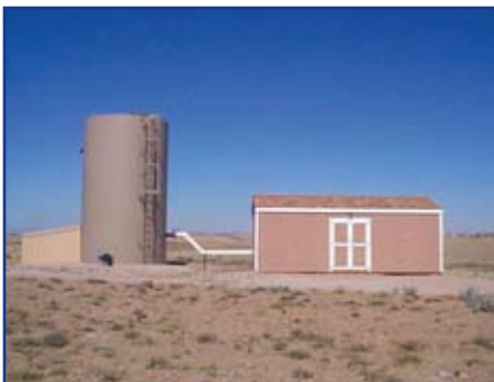
An injection facility, south of Gillette, showing the water tank and chlorination building. Photo courtesy of Marathon Oil.
